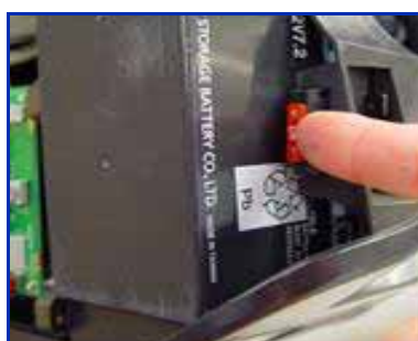
Fig. 3-3 Zekering in drive unit
