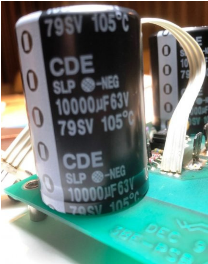
Figure 7. Replacement capacitor mounted.
